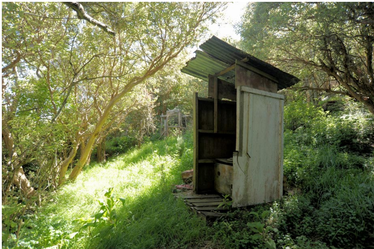
38 BEFORE: Room without a view – the original 'long drop' toilet now surrounded by native fuschia trees.
